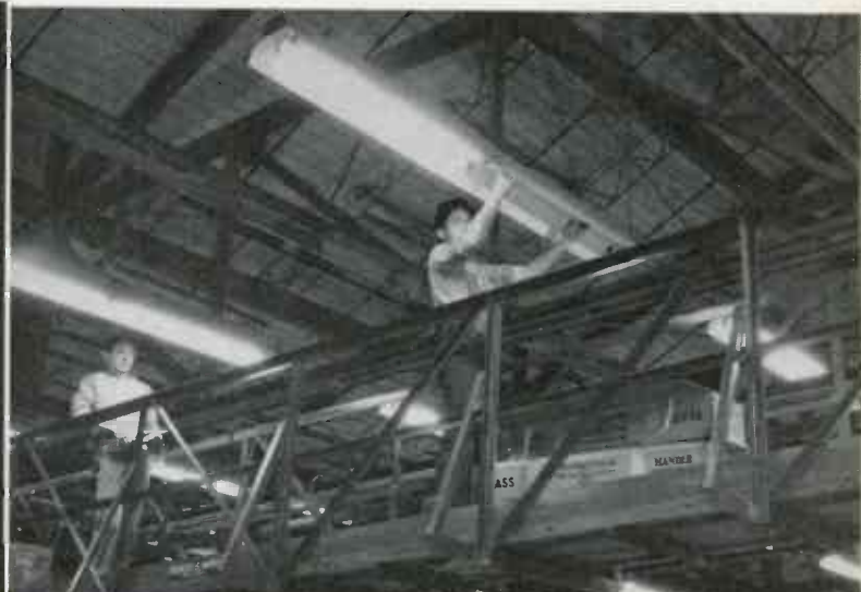
Servicing 18,000 fluorescents in Vega Aircraft, Burbank, Calif., plant, is facilitated by lamping bridge towed by monorail crane
